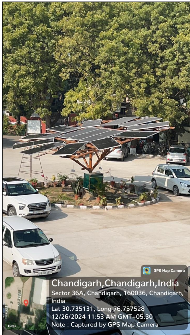
Solar Power Tree
