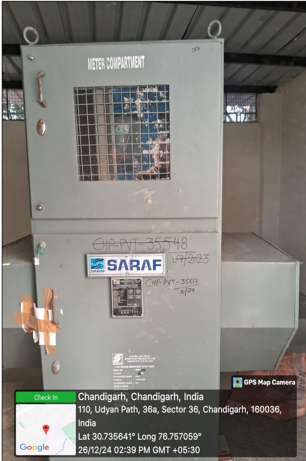
Net Metering Unit
