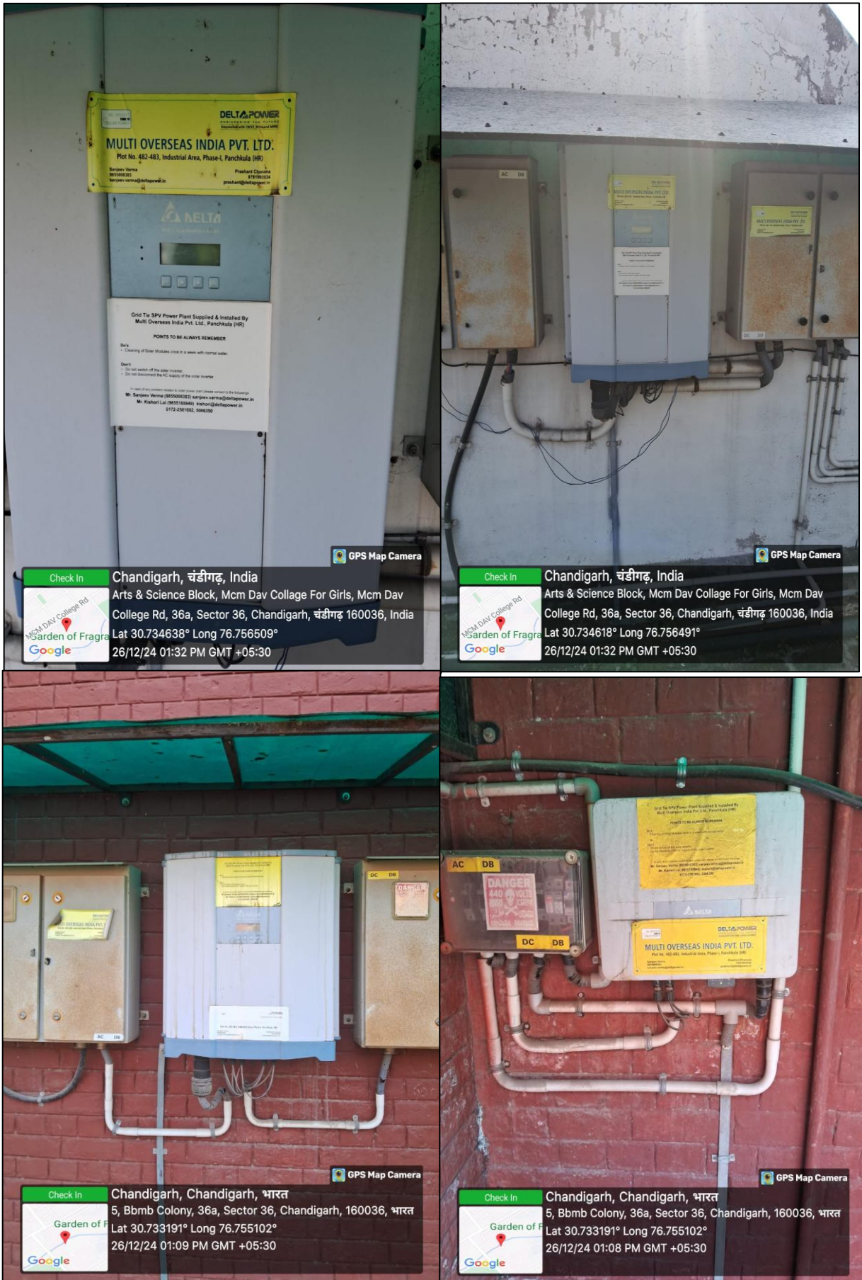
Wheeling to the Grid installed at solar roof tops
